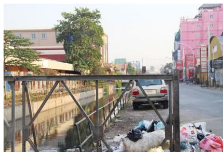
The Phnom Penh Post 28 April 2016 An area of the Boeung Trabek open sewer, where garbage spilling over into the canal is a normal occurrence.
